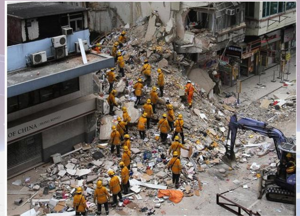
Hong-Kong building collapse (29th January 2010)
