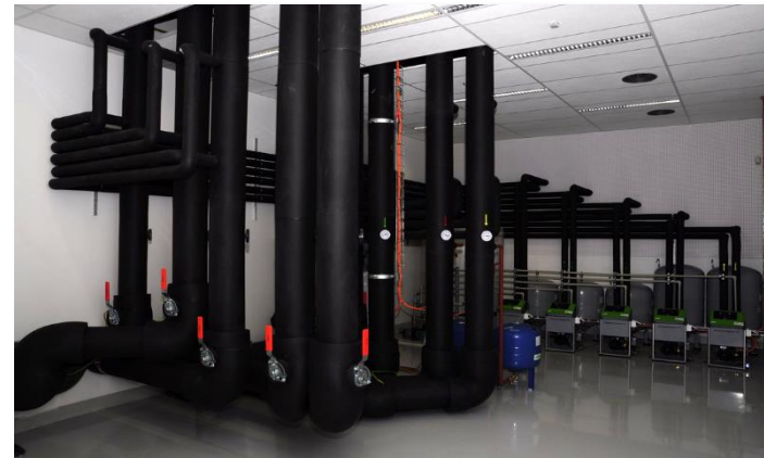
Cold and Hot water cooling
